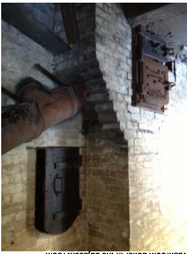
Washroom boiler in the adjacent room
