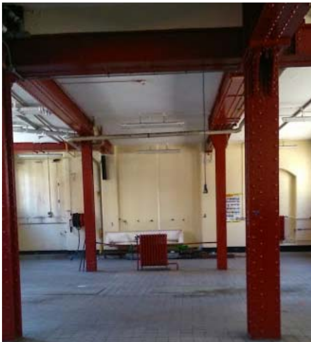
The appliance room
